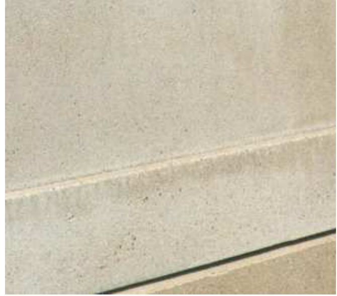
Efflorescence on a precast concrete panel. Source: CPCI
