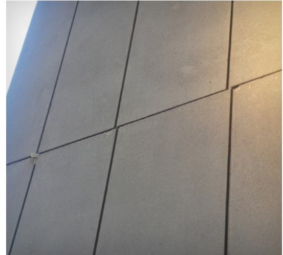
Misaligned panels—Alignment of panels directly impacts both aesthetics and joint sealing success.
