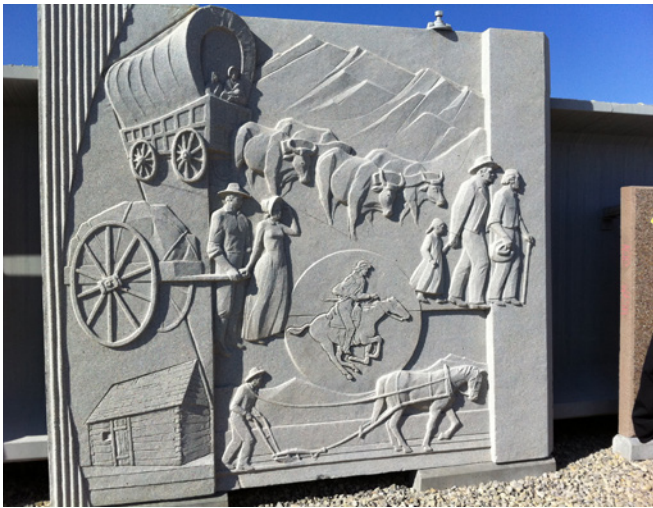
Form liners provide options for colour and texture. Source: M. E. Hachborn Engineering
