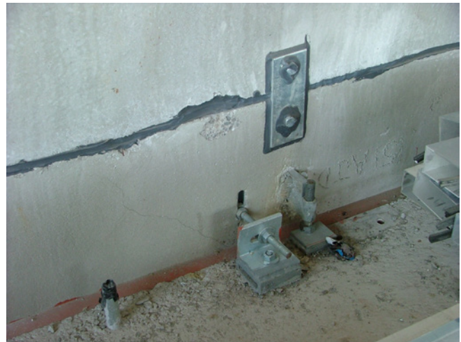
Interior-applied air/vapour sealant bead installed at panel joints and at panel connections. This is costly and not recommended. It is better to seal all joints from the exterior. Source: CPCI
