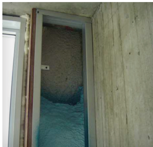
Spray polyurethane foam applied to the back face of a single wythe precast concrete wall panel. Source: Morrison Hershfield
