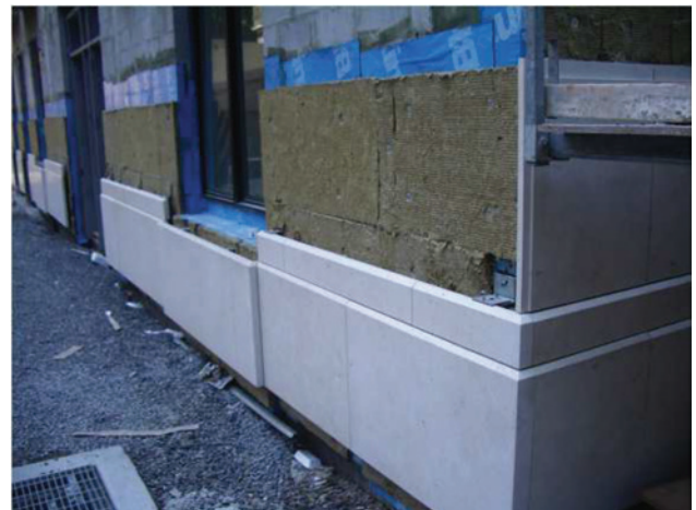
Handset precast panels installed in a drained wall system. This approach might be necessary for retrofit projects but is discouraged for new projects (See section 2.2.1). Image copyright RDH Building Science Inc., used with permission
