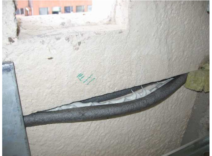
Loose backer rod. Backer rod too small for joint size, resulting in improper sealant application. Source: Morrison Hershfield
