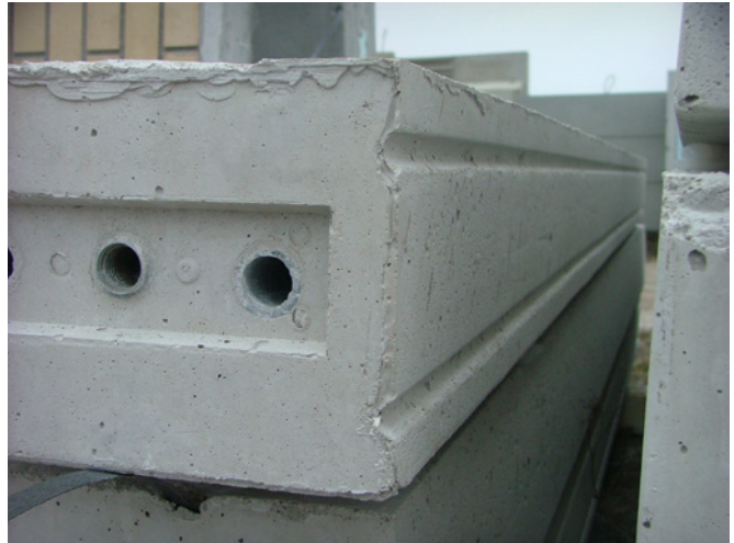
Drip Edge on a Precast Concrete Panel. Source: M. E. Hachborn Engineering
