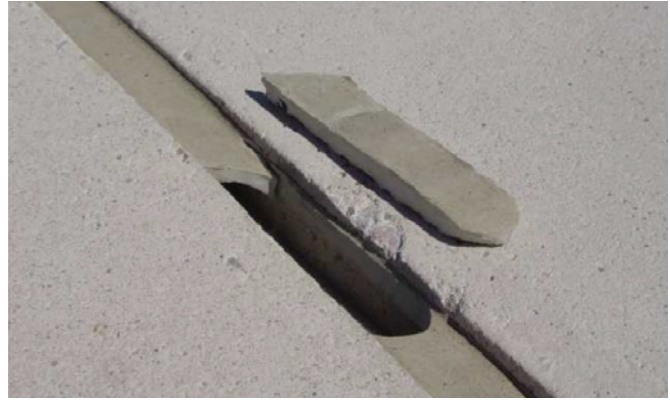
Sample testing of installed sealant to confirm proper dimensions. Source: Morrison Hershfield
