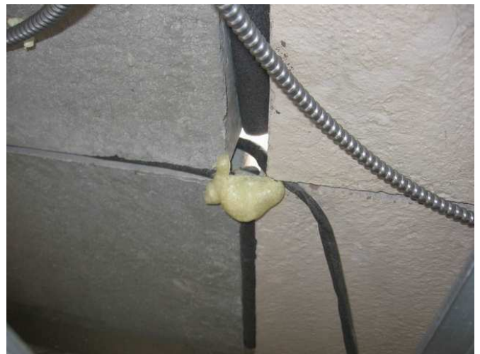
Loose backer rod. Backer rod too small for joint size. Note also that improper panel alignment has resulted in a wide range of panel joint sizes. Source: Morrison Hershfield
