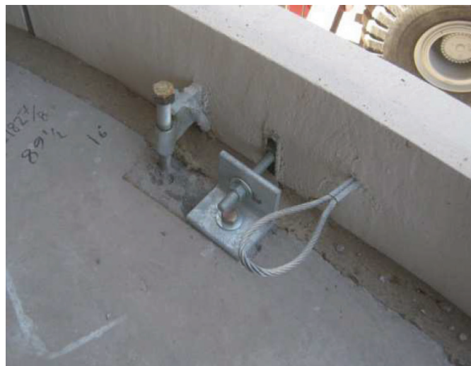
Gravity (vertical) load and lateral load connection, and lifting loop. Source: Morrison Hershfield
