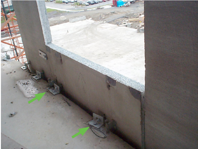
Eccentric (indicated by arrows) and lateral load connections. Source: Morrison Hershfield
