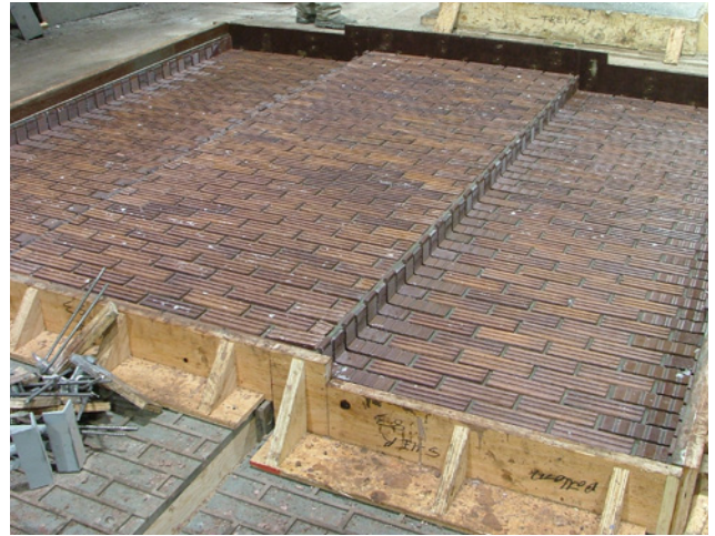
Masonry elements being placed in the rubber form liner, prior to concrete placement in the precast plant. Source: M. E. Hachborn Engineering
