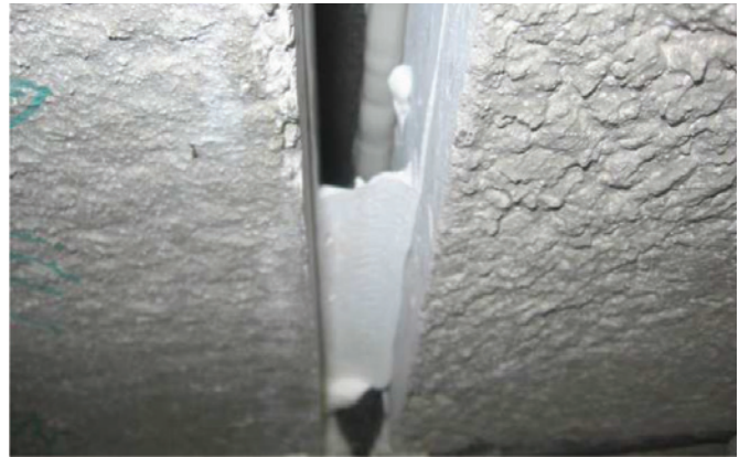
Sample testing of installed sealant to confirm proper dimensions. Note sealant bead is far too thin in this instance. Source: Morrison Hershfield
