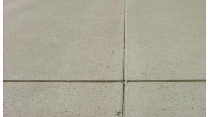
Unwanted shadow line at a panel butt joint. Source: CPCI
