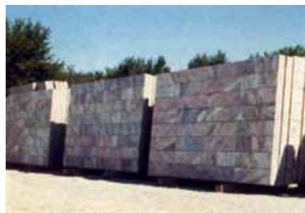
Architectural precast panels for the new wing of the Joslyn Art Museum, Omaha, Neb., are clad in Georgia marble to match the original stone building constructed in 1931. Labor and material cost were reduced using this system compared to traditional stone cladding systems.
