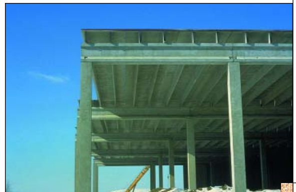
Long span double tees are ideal for food processing facilities.
