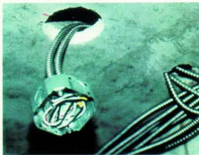
Cores used as raceways by electrical trades.
